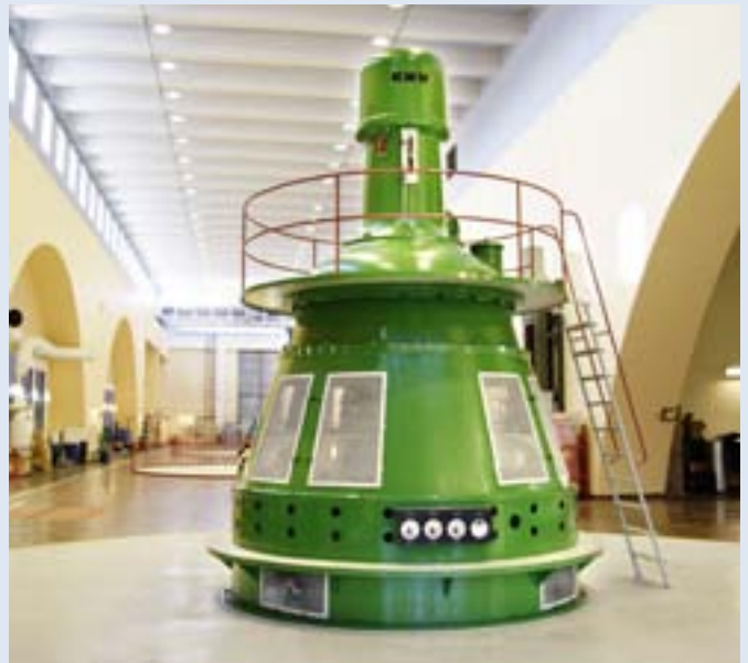
Midskogs Power Station Indalsalven.
