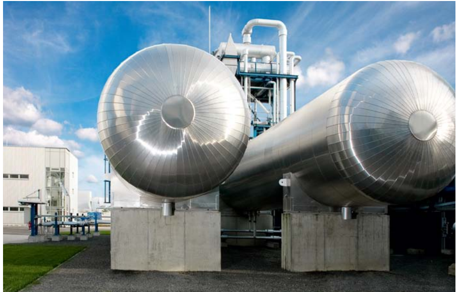
Carbon dioxide storage tanks at Schwarze Pumpe.
