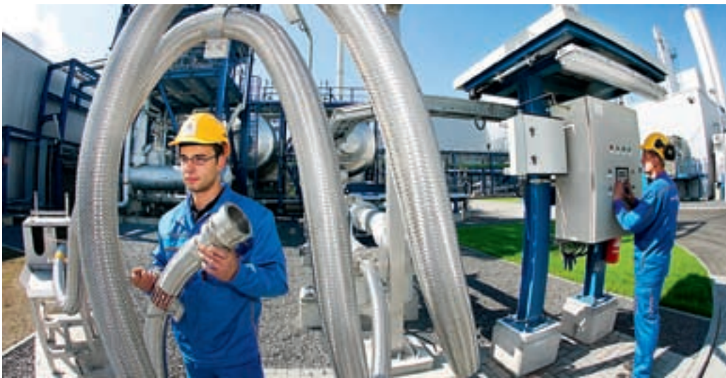
CCS pilot plant, Schwarze Pumpe, Germany.
