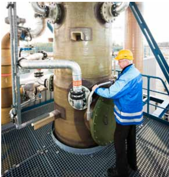
Operator besides the coal silo at the oxyfuel pilot plant in Schwarze Pumpe.
