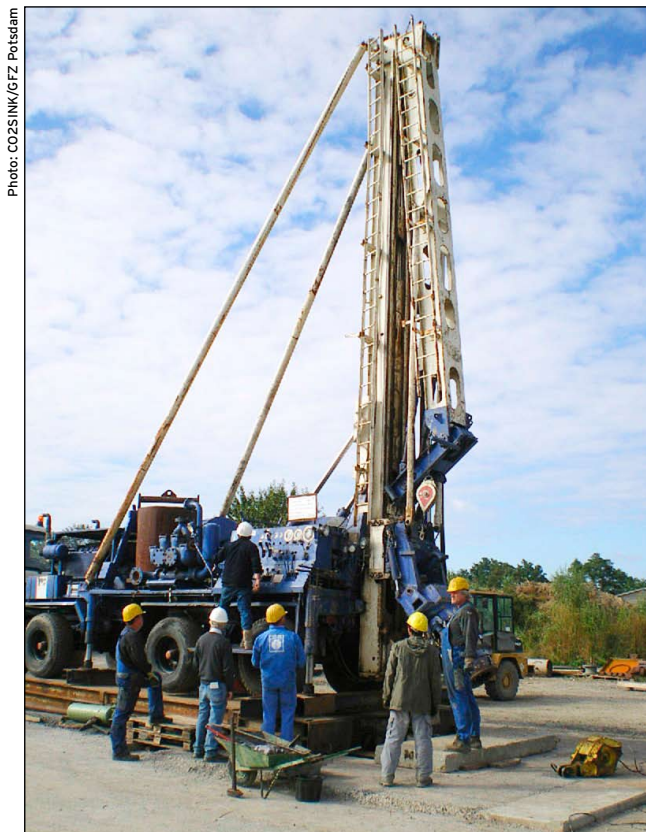
CO 2 SINK project: The small drilling rig is set up at Ketzin.
