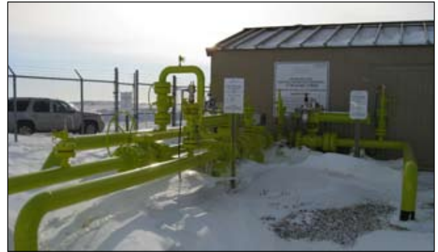
Weyburn central receiving terminal for CO 2 pipeline.
