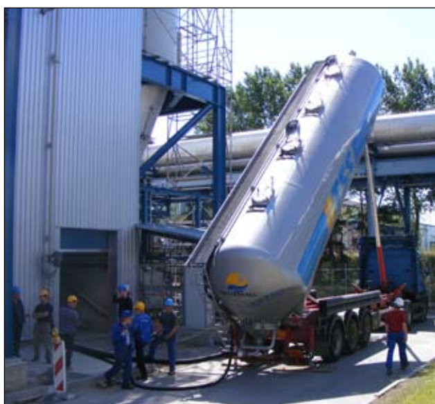
Pulverised and dried lignite is loaded in the fuel silos.
