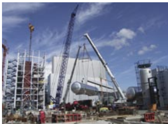
One of the CO 2 storage tanks is lifted into its final position after delivery
