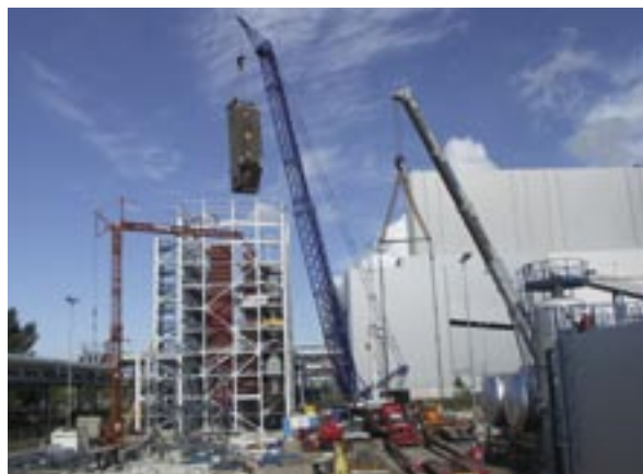
The furnace is lifted by a huge crane into the 25-metre high boiler house
