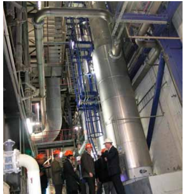
Esbjerg test facility in Denmark
